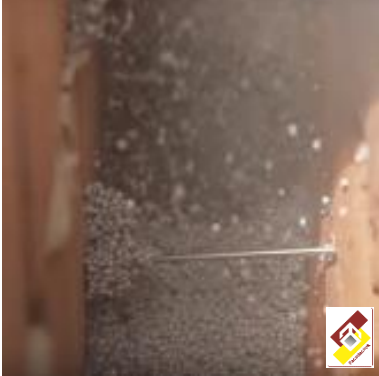
Wall cavity insulation
